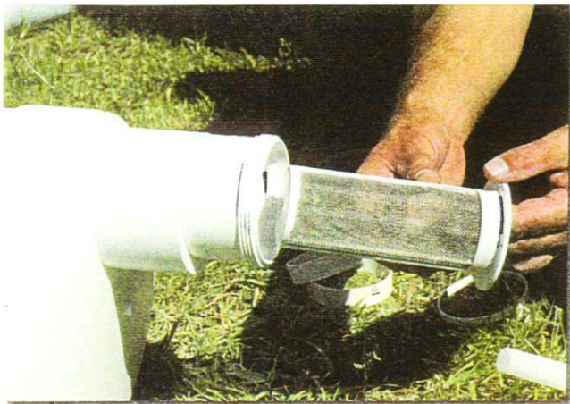
Mesh filter in first flush diverter.
