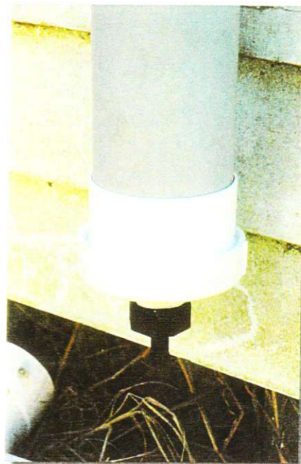
Drip filter in place.
